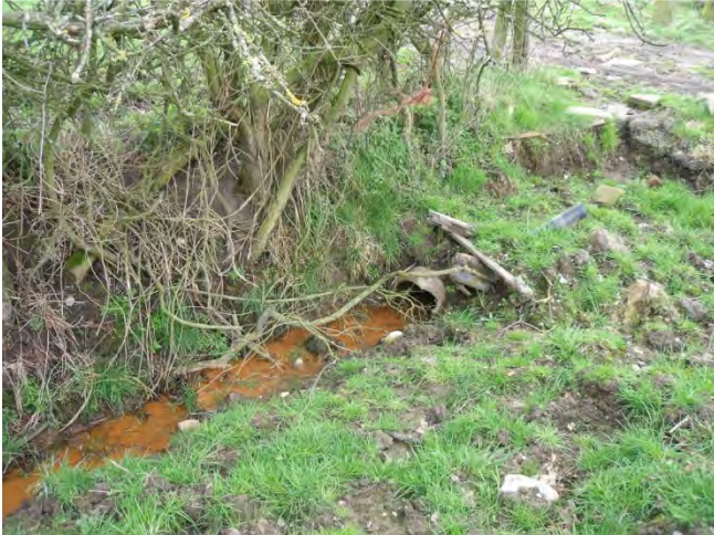
Photograph 15: View on outfall pipe to open land drain north of proposed highway.
